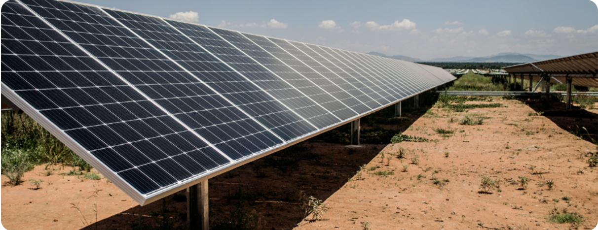
Santiago photovoltaic park, San Luis de Potosí, Mexico
